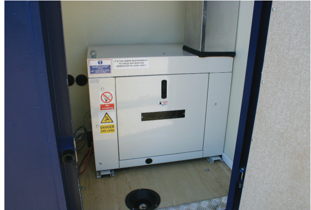
Welfare diesel generator
